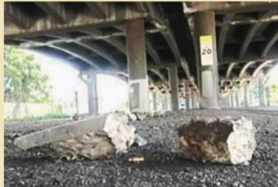
Falling pieces of concrete show a structurally deficient viaduct. This photo was taken on 46th Avenue under the viaduct
