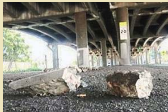
Falling pieces of concrete show a structurally deficient viaduct. The photo was taken on 46th Avenue under the viaduct.
